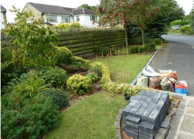
Marking the line of the path through the new section of garden before edging with bricks.
